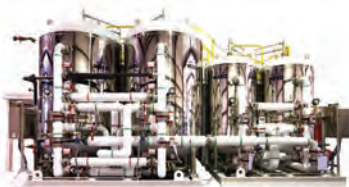
Carbon Filters & Softeners
