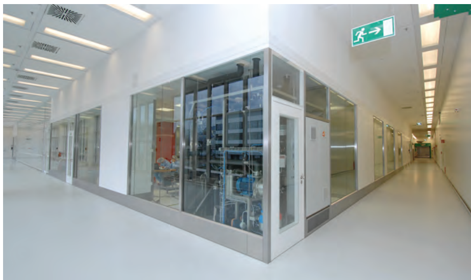
Surrounding corridor with view in the Aseptic Area 5.
