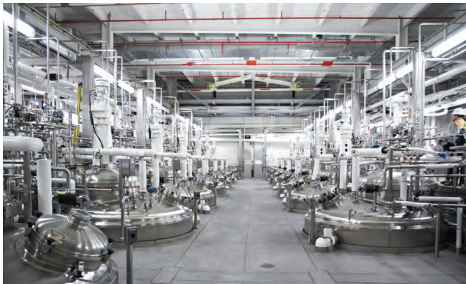
Completely closed processing allows the 12,000 L processing reactors to be placed in the unclassified technical core.
