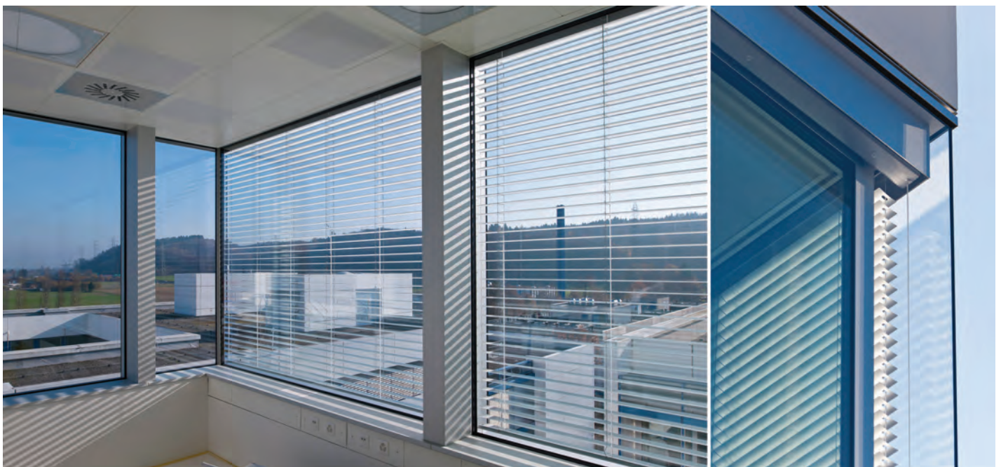
Close Cavity Façade (CCF) is composed of a triple glass thermal isolation layer on the inside and a simple glass pane on the outside.
