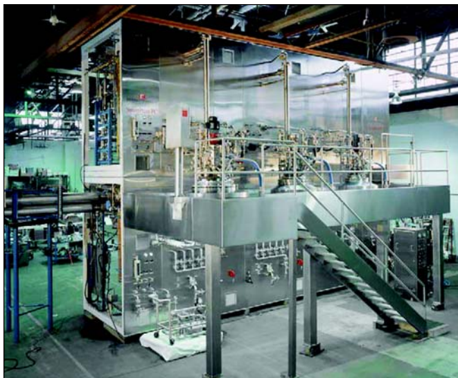
Figure 8. Modular Potent API unit undergoing Factory Acceptance Testing. 10
