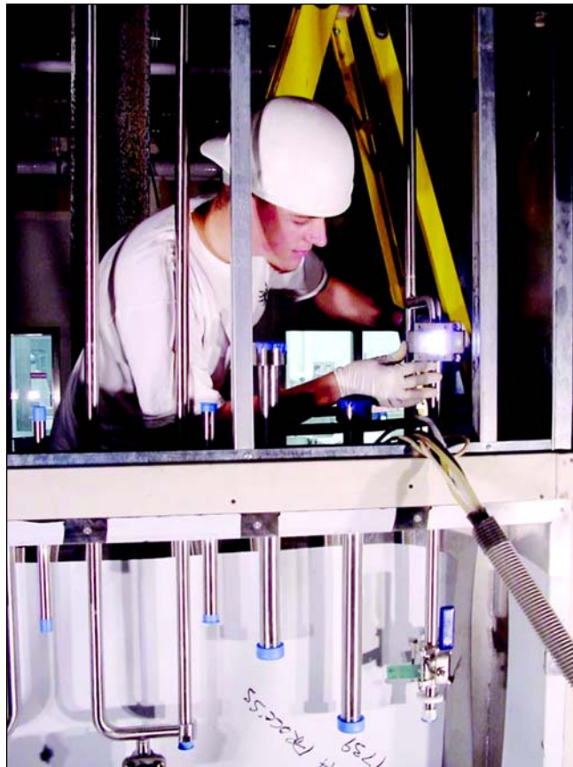
Figure 4. Orbital field welding of clean steam line to supply panel with a weld head. Welding operator is wearing gloves in compliance with contractor's SOP. The I.D. purge to this weld was twice the usual rate to compensate for a branch in the piping system. Photo courtesy of Sicom Inc.
